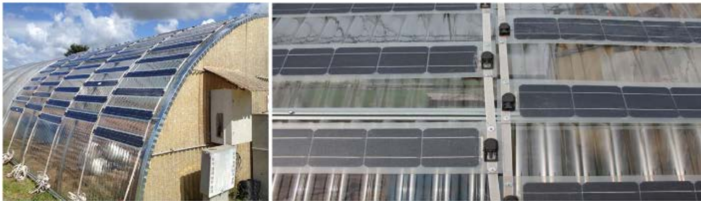
Fig. 2. Photo of PV panels installed on the greenhouse (left) and their detail (right). (Source: own elaboration).
